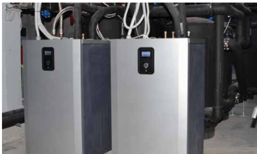
Heating room with two Mega ground-source heat pumps
