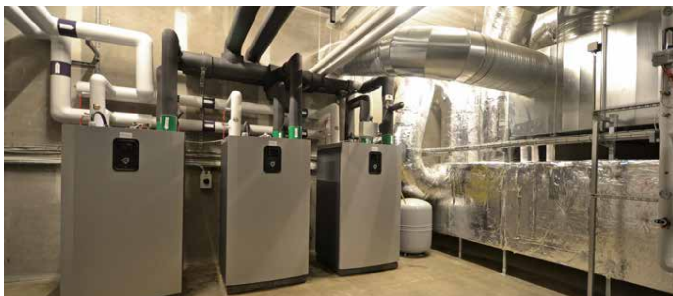
Heating room with Mega ground-source heat pumps
