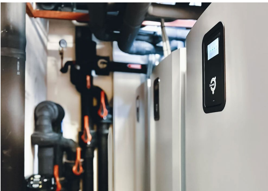
Three Thermia Mega L heat pumps in machinery room
